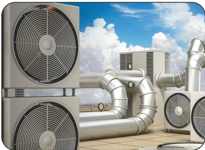
HVAC and Water Supply
